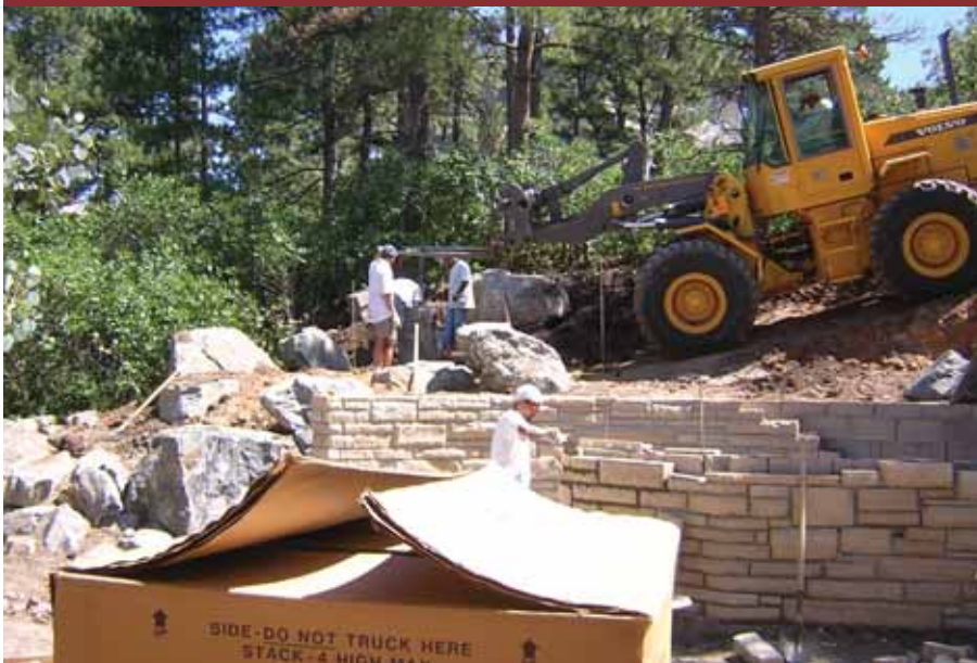
A front-end loader removed roughly 200 cubic yards of soil from the area that now houses the fireplace and spa.
